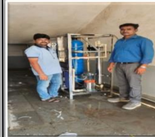
Establishment of RO Plant at Model School by Bala Vikasa
