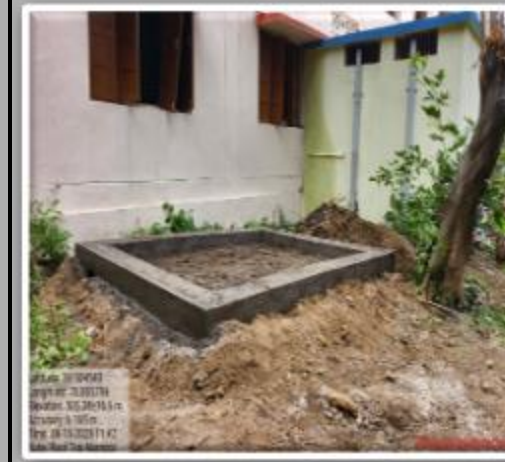
Roof Top Water Harvesting Structure at EMRS School
