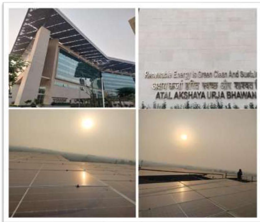
Ministry of New and Renewable Energy; 1 MW Rooftop Solar Power Plant at Urja Bhawan, New Delhi
