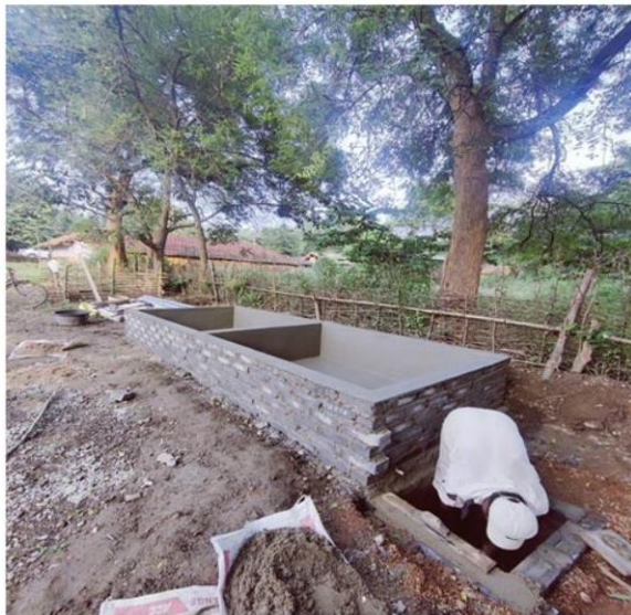
HCL Vermicompost plant- ICC unit, Ghatsila,
