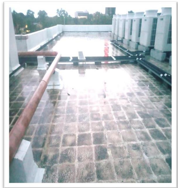
MECL Rainwater harvesting
