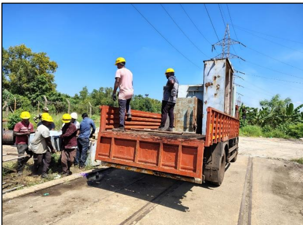
Metal scrap disposed of at Thermal Power Station – II, NLCIL, Chennai; Ministry of Coal
