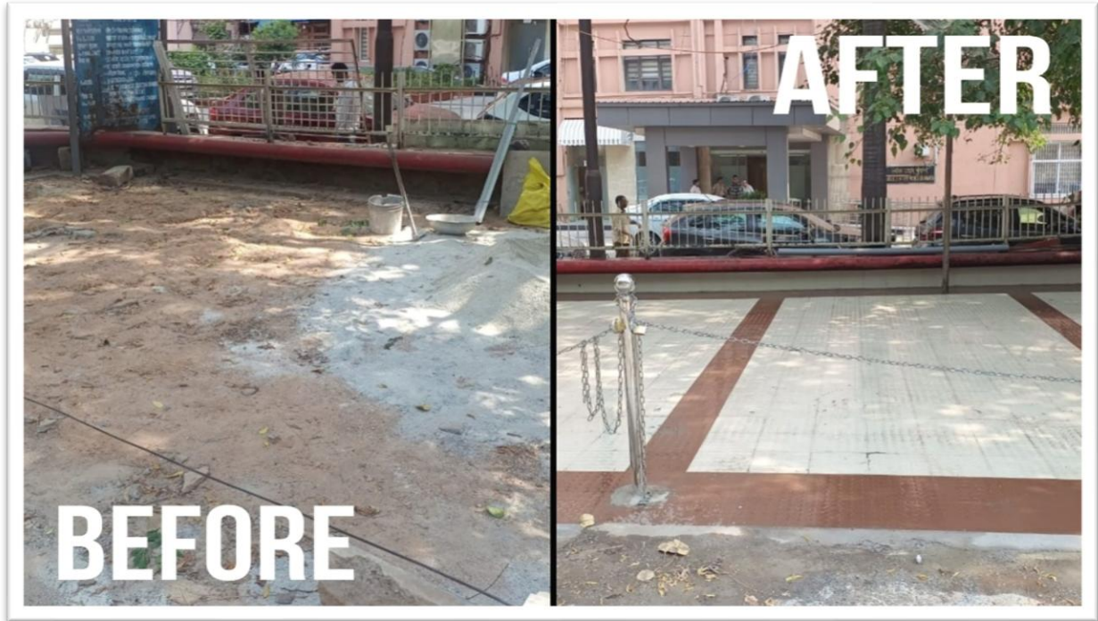
Enhanced Infrastructure at the Department of Public Enterprises (DPE) : From Uneven Ground to a Well-Paved and Organized Space: MoF
